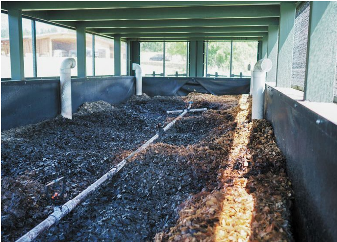
Inside a working BioFiltro unit, filled with worms. Photo provided by Biofiltro
